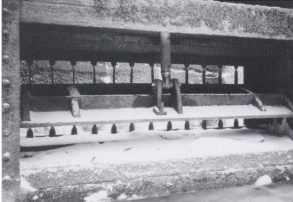
Figure B-7. Miter gate with butterfly valves
