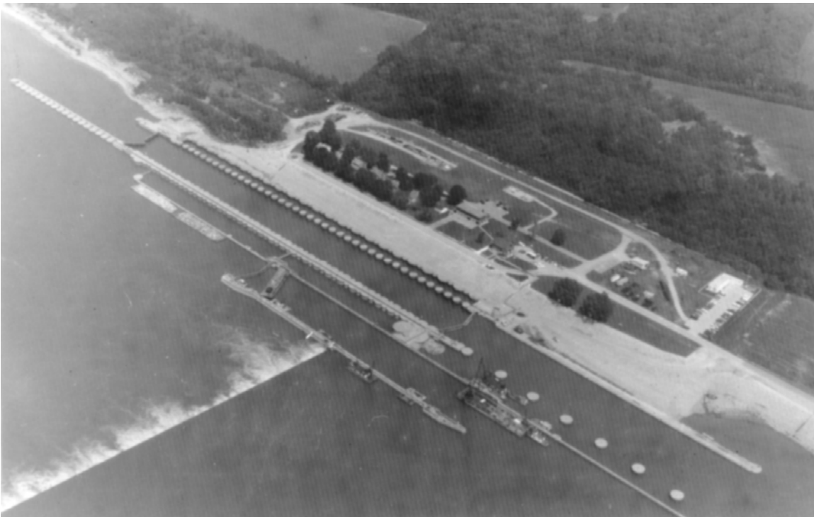
Figure 2-5. Temporary lock with cellular sheet pile. Lock and Dam No. 52, Ohio River, with design lift = 12 ft
